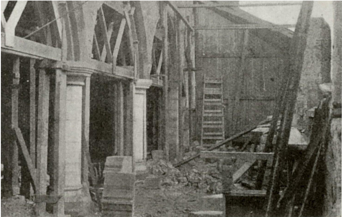
Work in progress on the north side of the building, looking west. The back of the partition built across the church can be seen.
