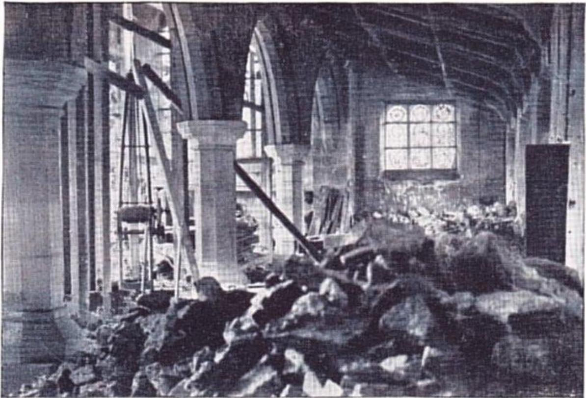
Three of the four rebuilt pillars and arches at the south-east of the church
